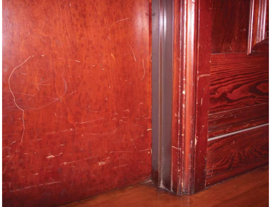
HEAVILY DAMAGED DOOR AND FRAME
